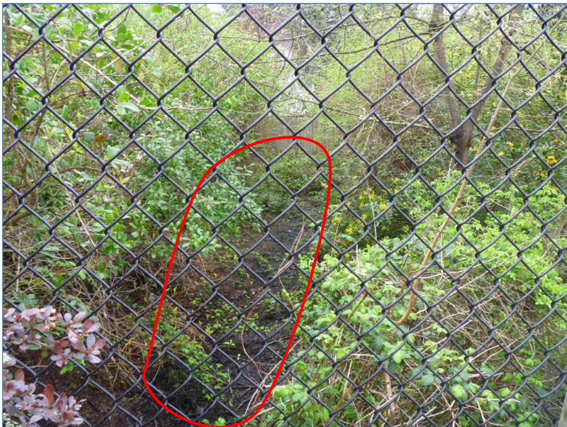
Figure 2. Possible Wetland PB01 pictured behind the fence (circled red). The visible portion of the area extends from a culvert (not pictured) to fence on the property line.
